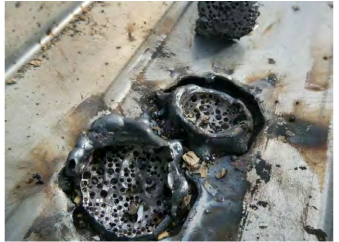
Fig. 9 • Faulty welds near a gap between sheet and girder.
