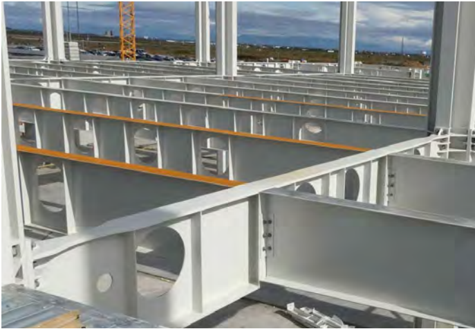
Fig. 8 • The coating on the upper flange must be removed, a thin layer of rust is harmless.
