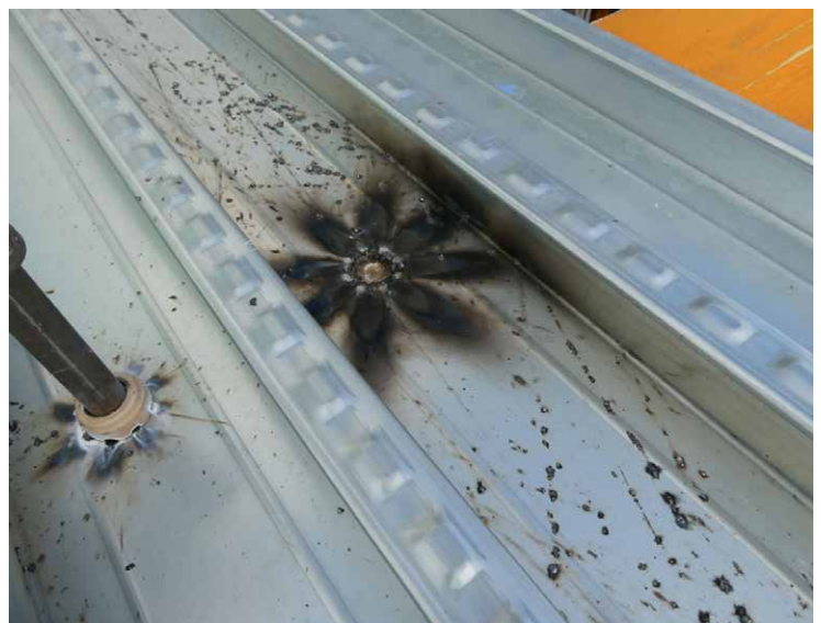
Fig. 6 • Attempted weld through a profiled sheet on a coated upper flange.
