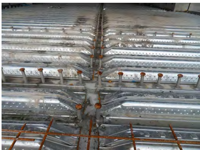
Fig. 2 • The openings of the profiled sheets have been closed by pressing them down.
